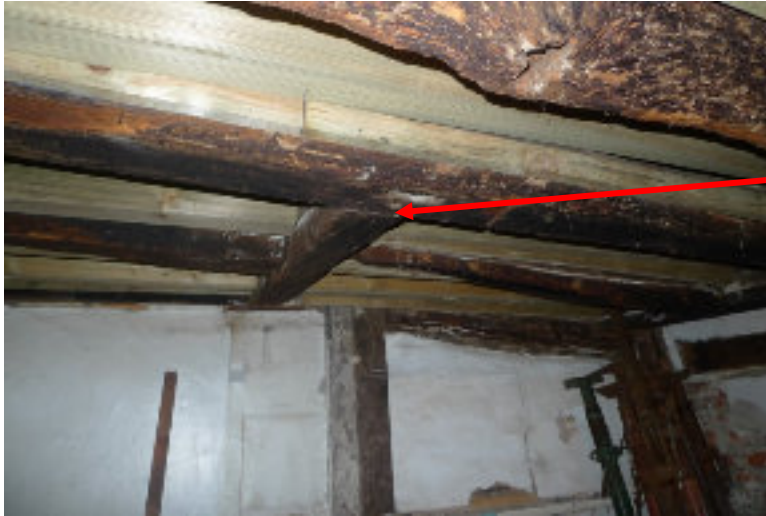
FIG. 8 Framing in floor in bay EF showing the trimmer for a staircase in the rear corner of the bay. This would have originally allowed a space in the corner for a ladder stair to access the first floor.
