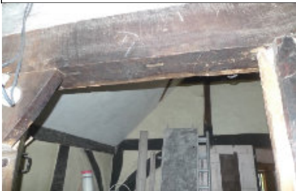
FIG. 9 Tie beam in Truss D. The stave holes in its soffit were to form a wall. This means there was no way through the smoke bay suggesting there was no further bay beyond the smoke bay.
