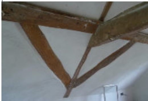
Below: The straight windbraces and clasped purlin of the cross wing roof.
