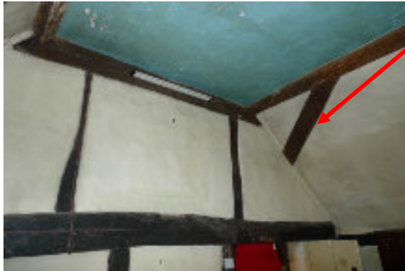
FIG. 6 Straight windbrace between the clasped purlin and the rafter at post D
